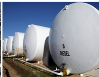
Above-ground and Underground Storage Tanks
